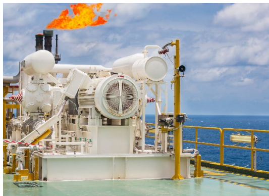
Vapor Recovery Unit (VRU)
