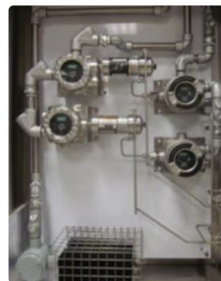
TriGas X5000 System (Inside Enclosure)
