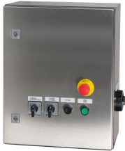
Motor control cabinet
